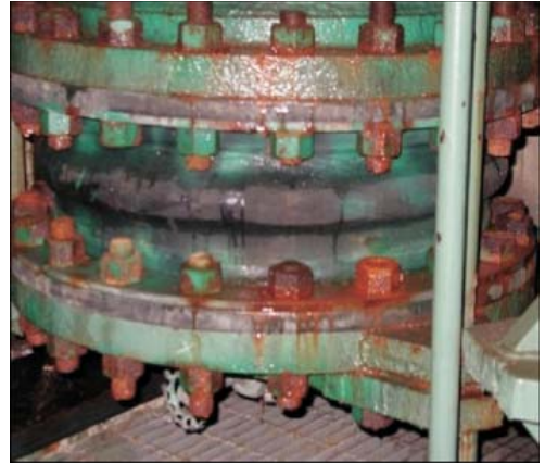
Figure 3. Leaking Expansion Joint
