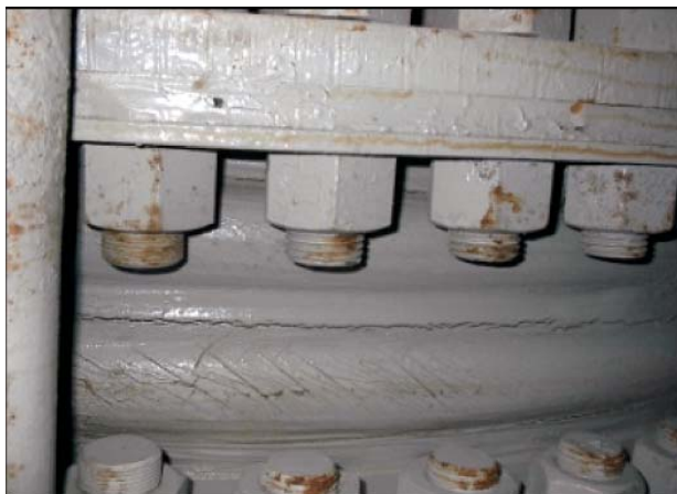
Figure 1. Typical Expansion Joint Surface Cracking
