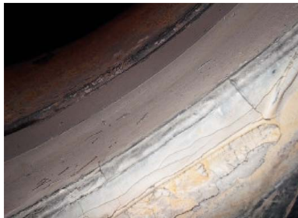
Figure 2. Expansion Joint Surface Delamination
